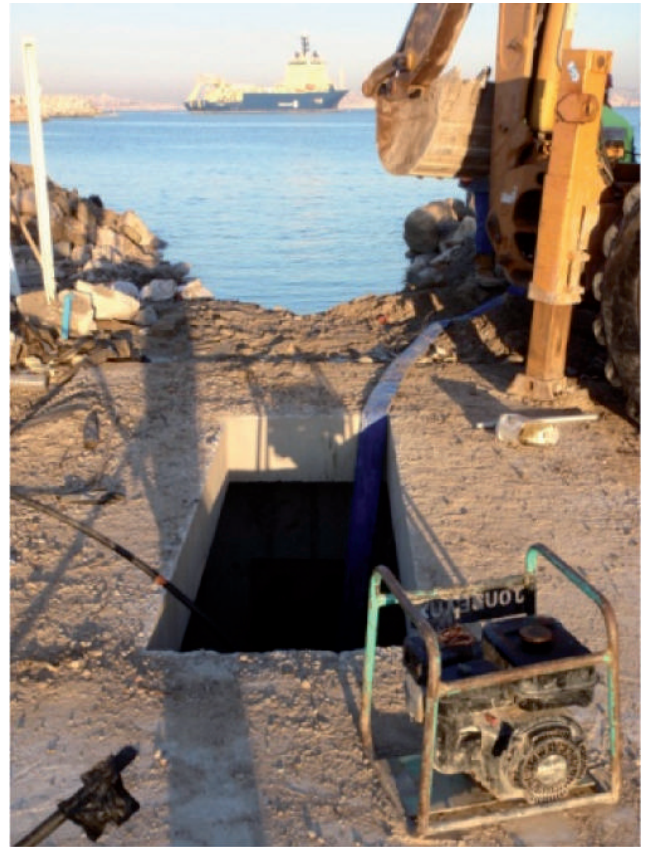
Figure 12. BMH for a telecommunications cable entry in Marseille (France).
