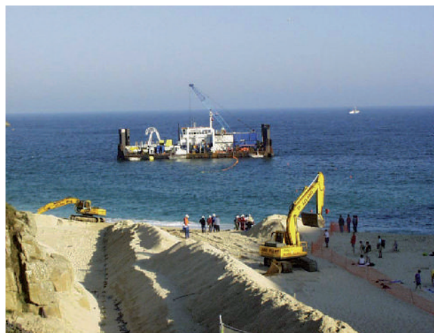
Figure 40. Submarine cable installation works in the coastal zone from BMH to low water mark. Source: www.ldravocean.fr.
